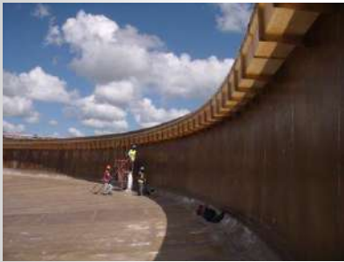
Clarifier liner and internals
