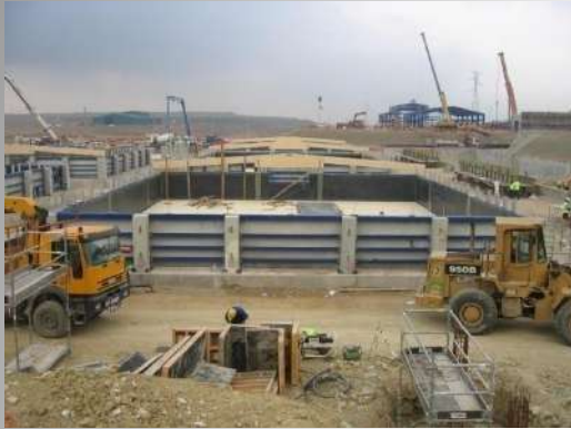
Settler tanks - Spain
