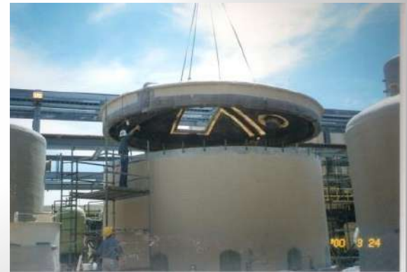
25' dia. FRP clarifier
