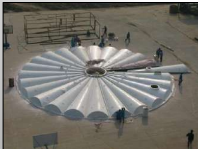
60' dia. clarifier cover
