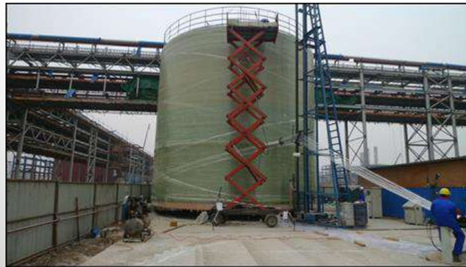
Field wound process water tank
