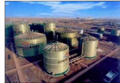
Tank farm of field wound tanks
