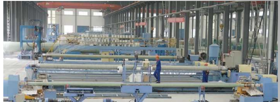
Piping systems for SNC Lavalin, Serbia acid plant
